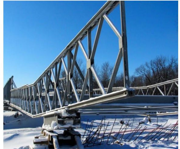
2015 Algonquin detour bridge project for Ministère des Transports Quebec on Autoroute 40, near Berthierville
