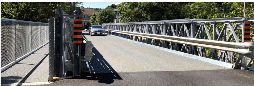
Temporary detour bridges in use at Marlborough Wood (top) and Belmont on the Arm (bottom)
