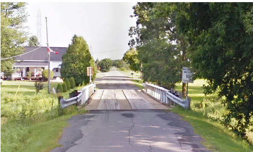
The original bridge was ordered closed due to "failing in key areas"
